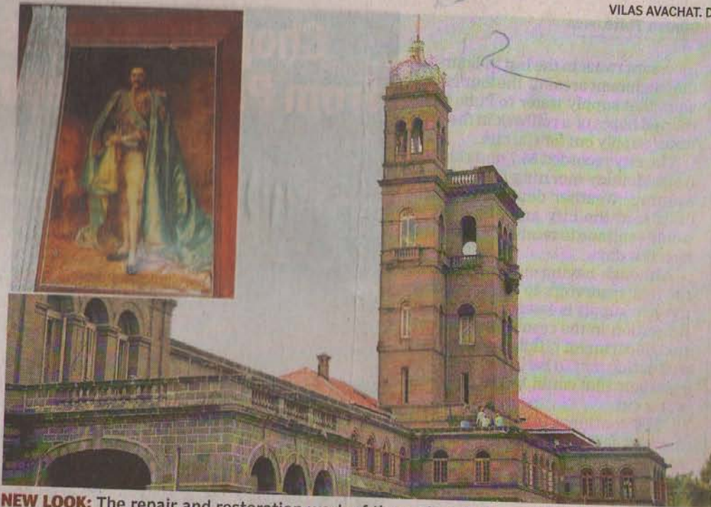
NEW LOOK: The repair and restoration work of the main building of the University of Pune is gaining momentum as the roof restoration work was completed recently; (inset) a British era painting among others was damaged due to sipping water from the roof.
